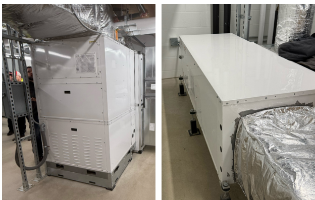
The design team selected multiple Versatec 500 and 700 water source heat pumps in both horizontal and vertical configurations.
