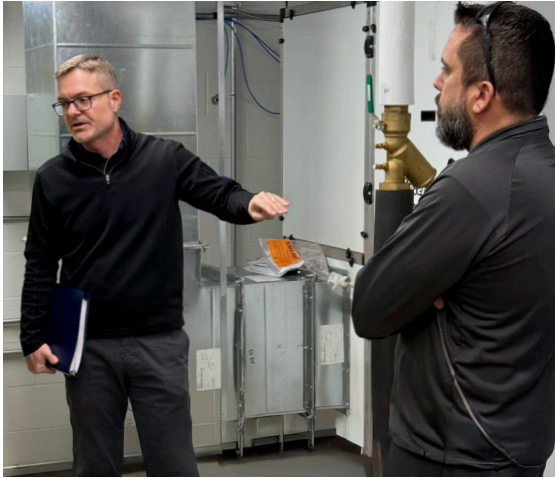
JP Heisserer reviews the details of the McMillen Family Pavilion's geothermal system.
