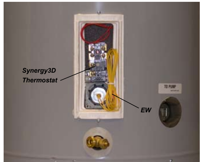
Yellow thermistor wires connected to TB (3 & 4) on EW control board
